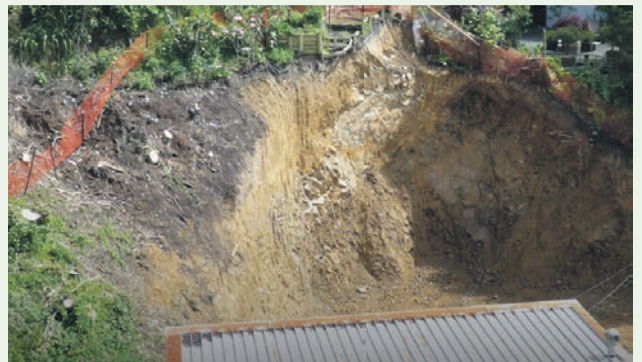
Townhouse excavation caused boundary problems in Mt Cook.
