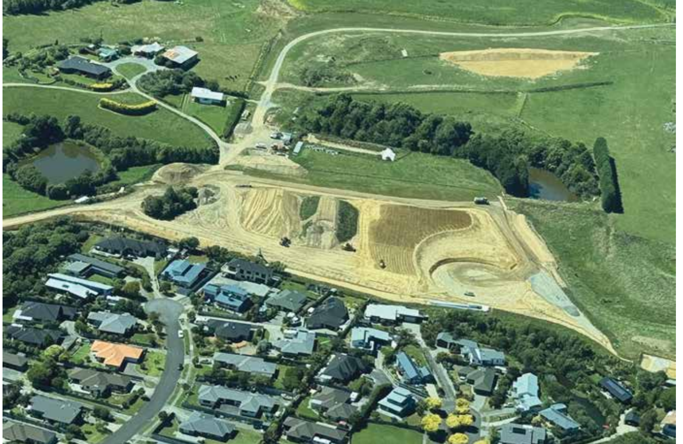
An aerial photo showing the reservoir site in early March. The reservoir itself will be built in the circular space at the bottom right of the earthworks.
