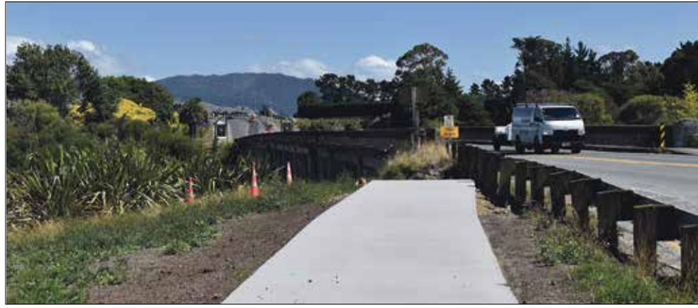
The old Ōtaki River bridge, with a new path waiting to connect to the “clip-on”. Photo Ōtaki Today
