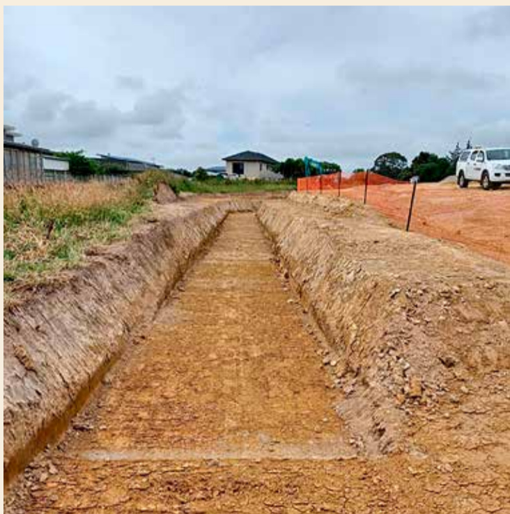
The trench for the pipes from the reservoir to Te Manuao Road.
