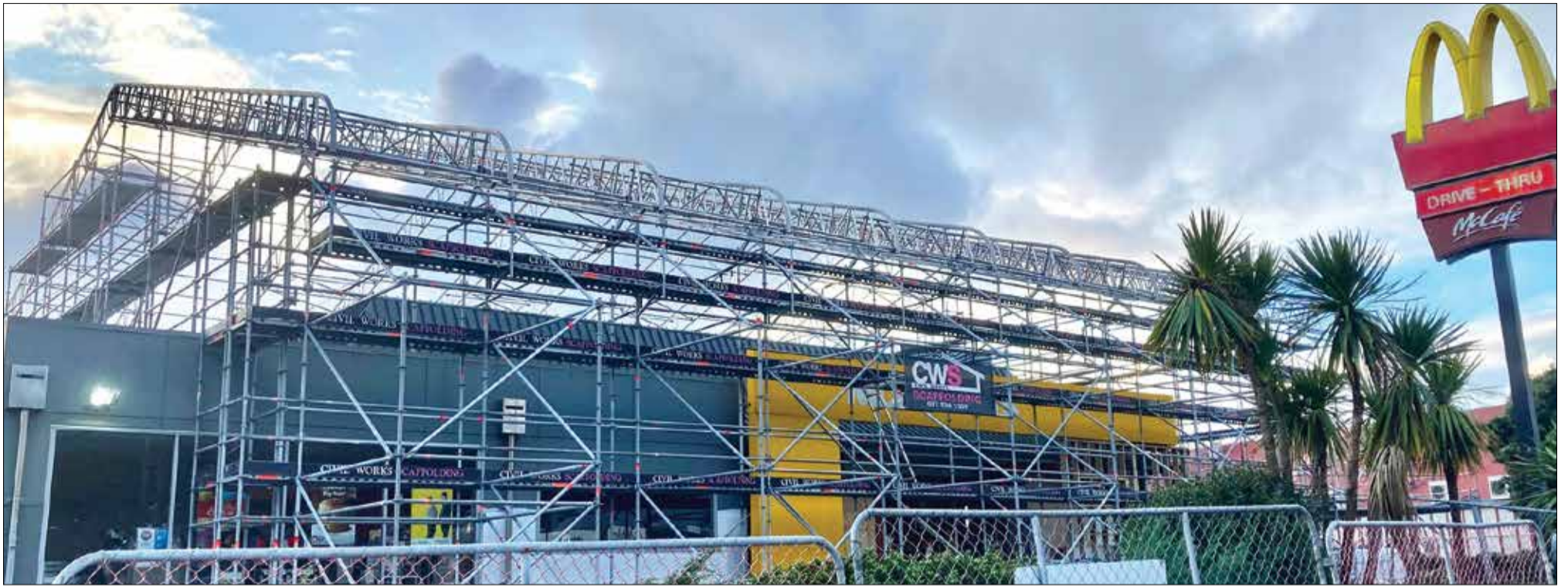
Civil Works Scaffolding in use on a Paraparaumu site. CWS has scaffold solutions for large building sites such as this, and for small local home owners.
