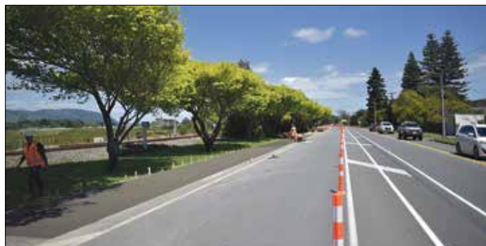
Work on the shared pathway north of the bridge. Photos Ōtaki Today
