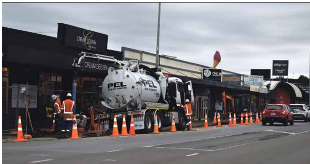
PIPES: Works to install a gas line to a new pizza store blocked car parks at some highway shops for several days late last month.
