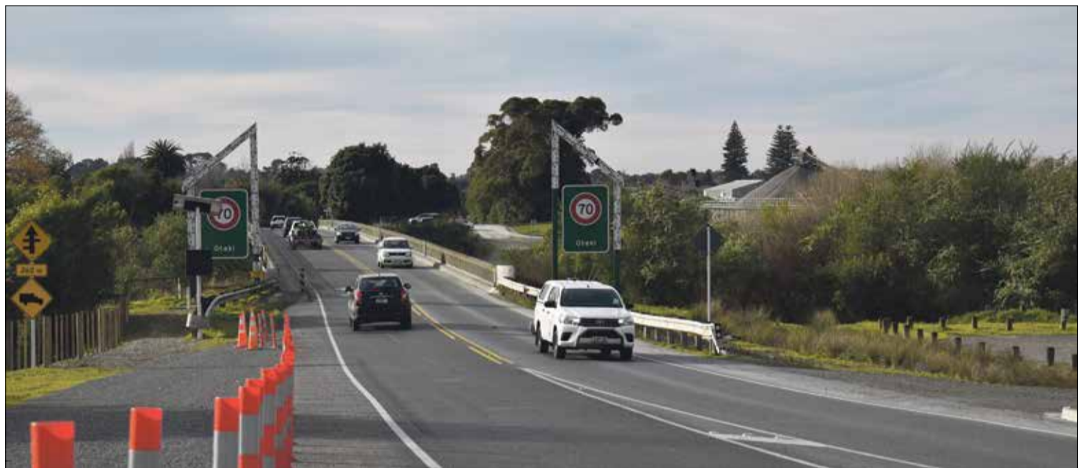
The Ōtaki River bridge on the old main highway, where works later this month and during summer will require partial closure.
